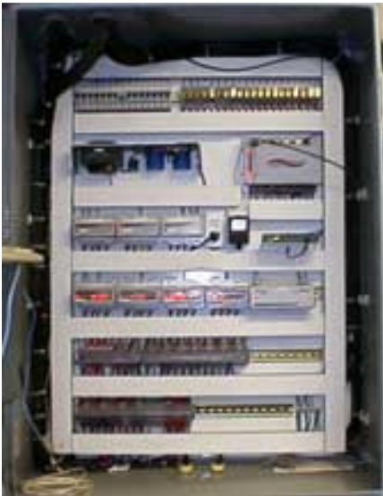
Figure 5 Typical Ethernet-based controller panel
